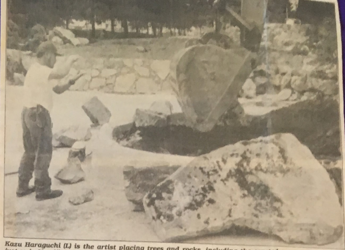
Kazu Haraguchi (L) is the artist placing trees and rocks, including the coveted moss-covered ones, just so in Momiji Garden, under construction at the PNE. Rob Truyst photo
